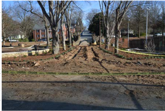
Renovations of the maple allee' began in late January. Photos by M. Lively
